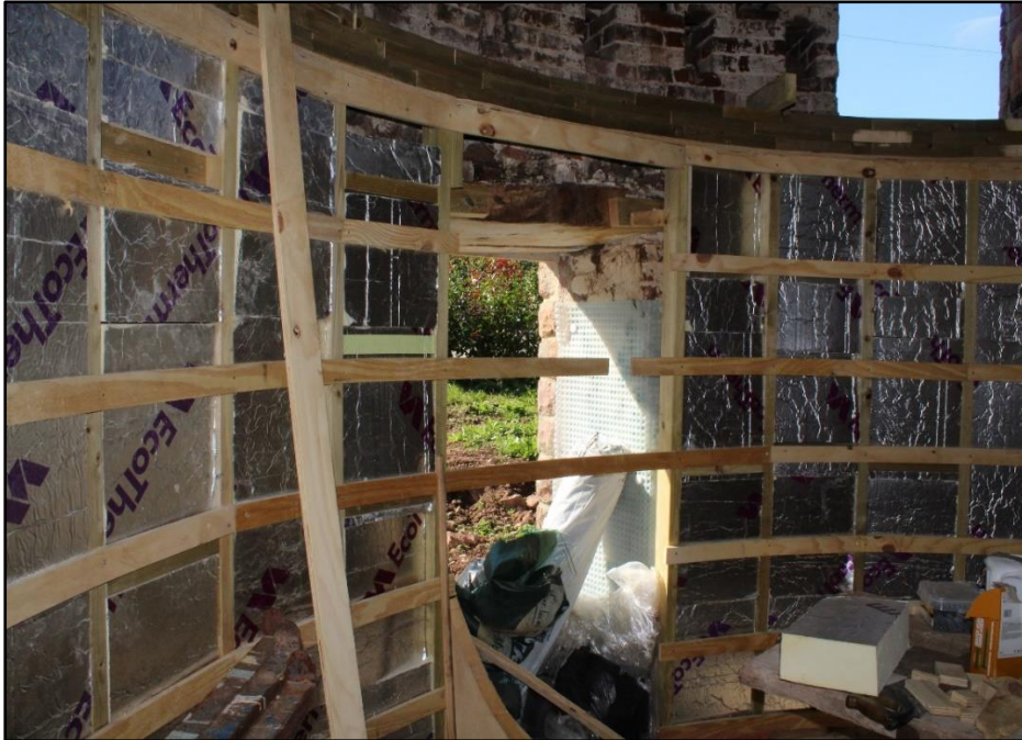
Figure 1: Upgrading of solid walls with modern non-vapour permeable tanking membranes and high density polyisocyanurate insulation board (Source: Gwynne 2018).
