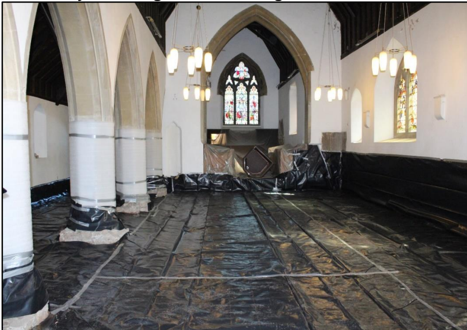
Figure 2: Polythene damp proof membrane laid over the floor area and dressed up walls (to hide existing rising damp) ready to receive 100mm thick high-density polyurethane insulation board, 100mm dense concrete slab and ceramic tiles (Source: Gwynne, 2019).
