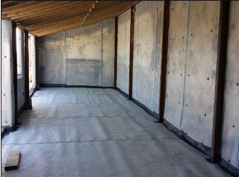
Figure 3: Water proof tanking system fixed to top of original floor and internal face of solid stone walls to prevent damp ingress ready to receive a high density polyisocyanurate insulation board and concrete slab to floor and same insulation fixed between timber stud walls with vapour checked plaster board fixed around the inside perimeter (Source: Gwynne, 2018).
