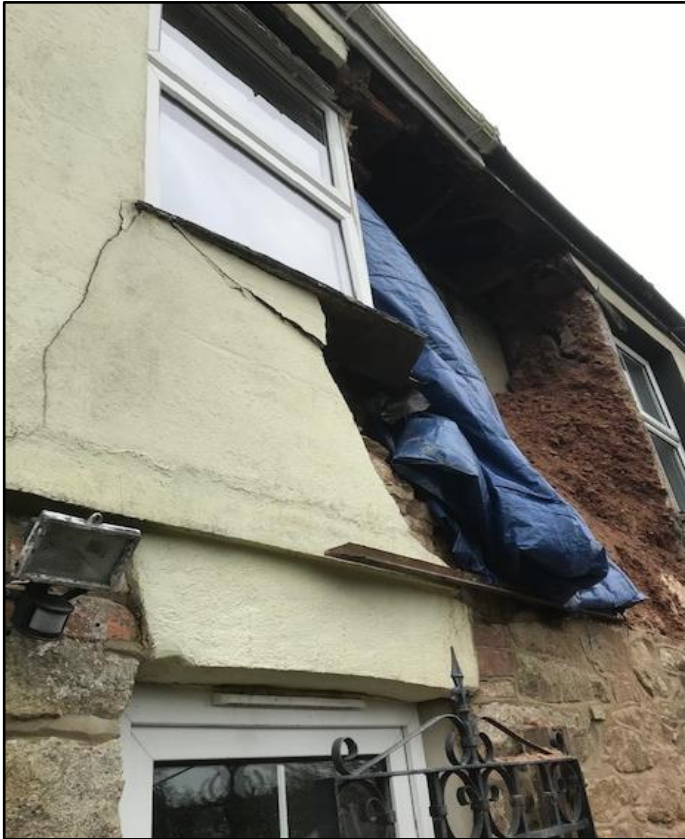
Figure 5: Collapse of the cob wall caused by water trapped behind hard cement render (Source: Gwynne, 2019).
