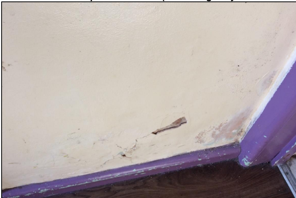
Figure 4: Rising damp and Crypto fluorescence pushing off hard gypsum plaster (Source: Gwynne, 2017).
